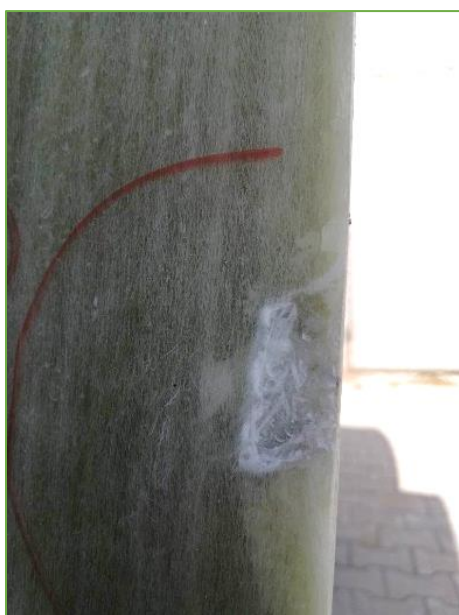
Figure 23: Can be repaired on site surface damage
