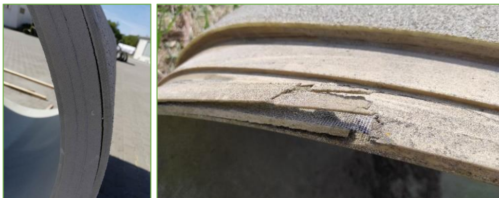
Figure 24: Structural defects that cannot be repaired on site
