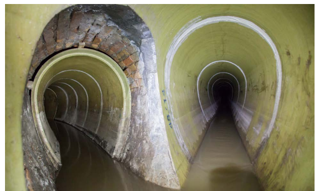
Junction of pipes
